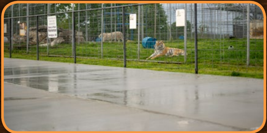
Shortly before we had to temporarily close due to COVID-19 we poured concrete in our discovery area, making it easier for everyone to navigate.
