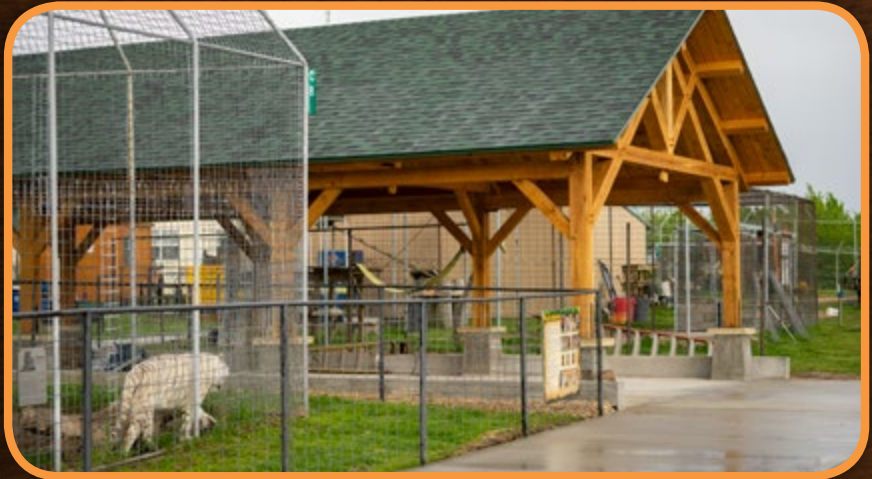
We also had begun construction of a new Pavilion to provide shade, a gathering area, and an outdoor educational area near the big cats.
